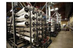
Photo: Reverse Osmosis Unit
