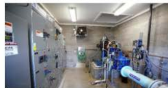
Photo: Well Pump House
